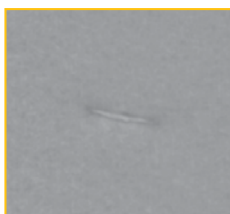
Broken Coating Layer
