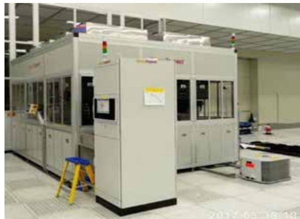
Offline ParticleInspect Solution in Mini-Environment in a Cleanroom Production Site
